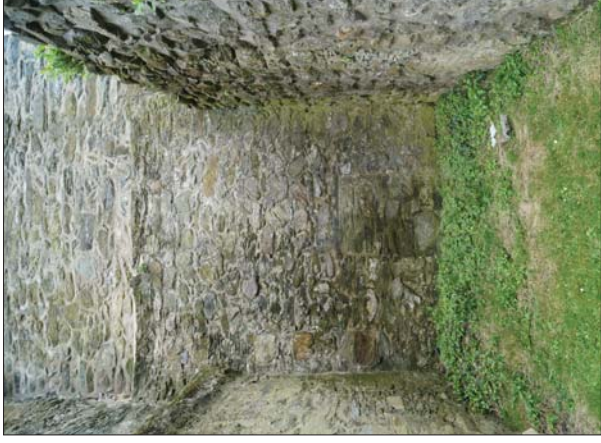
Plate 30. Blocked Opening At Base of Church Tower
