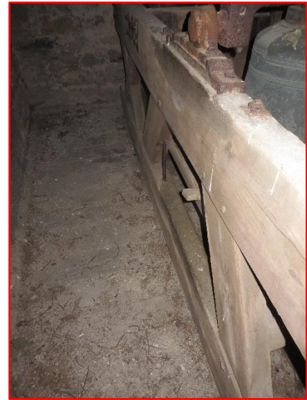
OUTSIDE OF TREBLE FRAME SIDE SHOWING INCLINED BRACES, HEAD, CILL AND X-BRACE ACROSS END OF SECOND PIT
